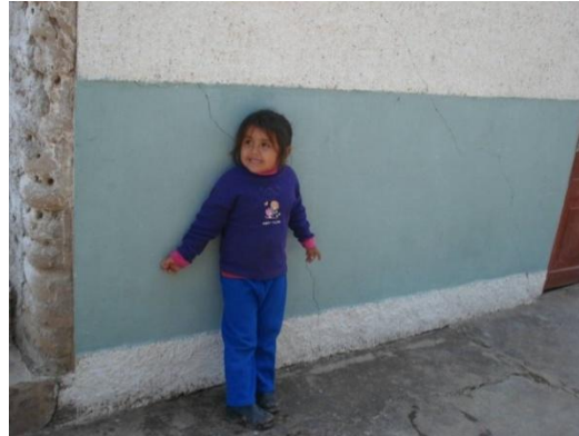
Figure 1: Girl in a place of risk from the damaged building, Peru. Photo: Soluciones Prácticas.
