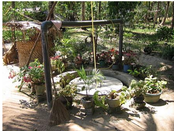
Figure 8: Biogas plant installed in garden in Sri Lanka Photo: © Steven Hunt/Practical Action
