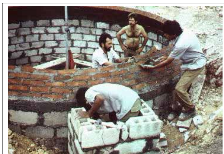
Figure 17: Construction of the dome for a 30 m 3 digester in Cuba Photo: Krämer (TBW)
