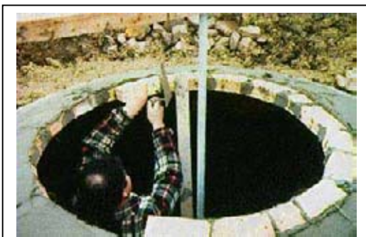
Figure 3: Fixed-dome plant in Tunisia. The final layers of the masonry structure are being fixed.
