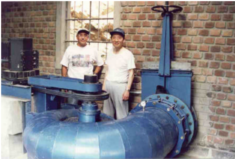
Fig. 7 Axial turbine after final assembly
